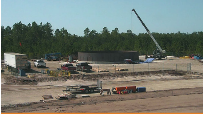
The Maxville LNG facility being built by Eagle LNG Partners LLC is expected to be fully operational by mid-2017.
