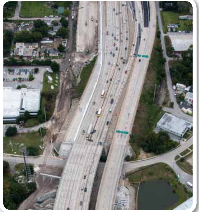
Aerial view of the Interstate 95 Overland Bridge construction project, which is designed to improve traffic flow along the I-95 corridor just south of the Fuller Warren Bridge in Jacksonville.
