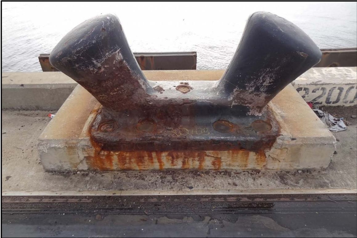
PHOTO 2-20 Mooring bollard with 25 percent coating loss and moderate corrosion and pitting.
