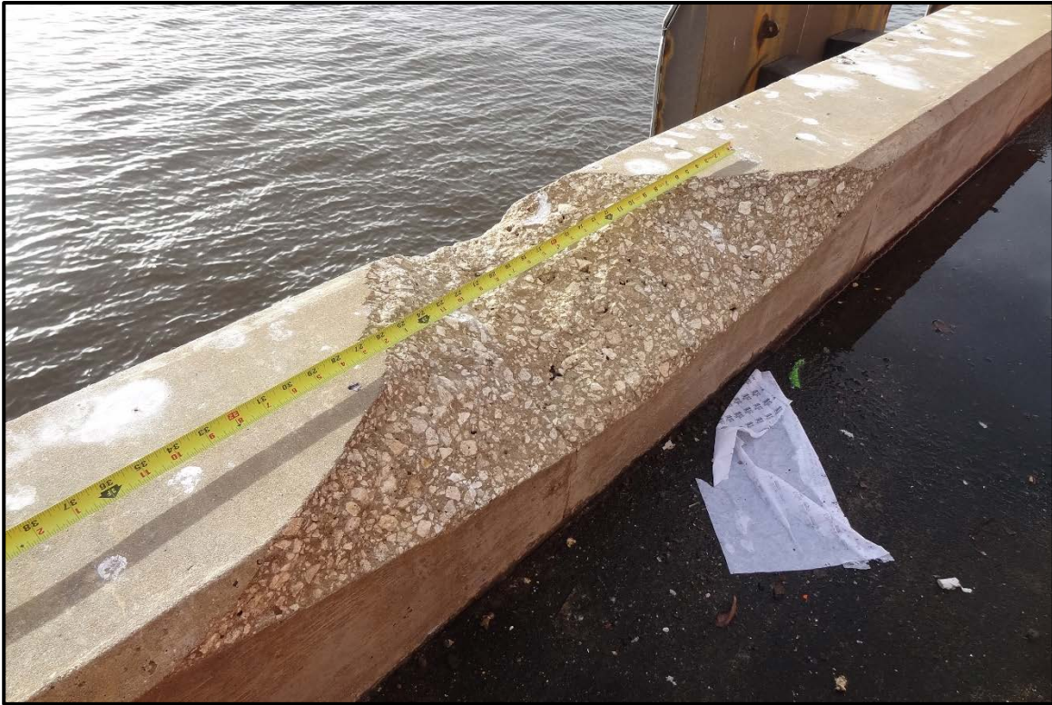
PHOTO 2-18 Mechanical spall in concrete curb at Station 25+40.
