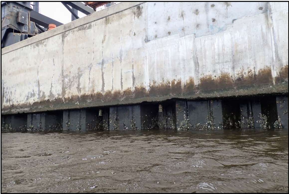
PHOTO 2-17 Capping beam with typical mechanical spalling on the bottom corner.
