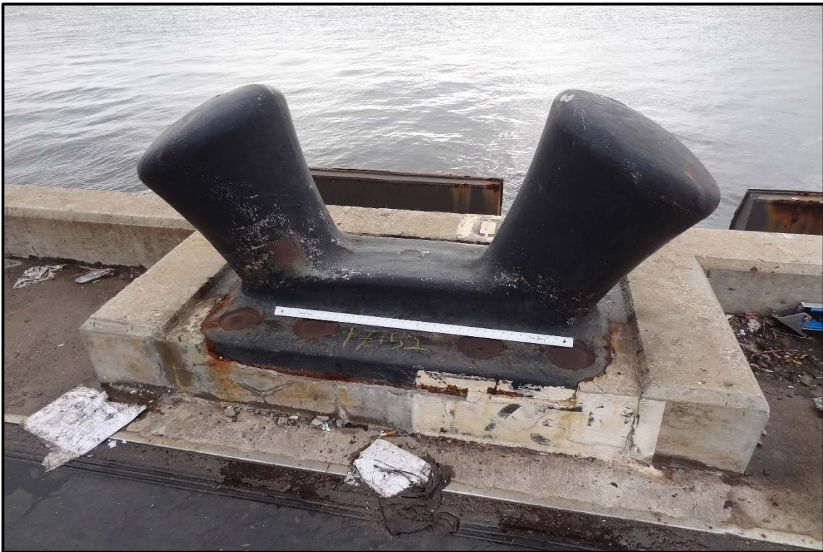
PHOTO 2-19 Typical mooring bollard with 5 percent coating loss and minor corrosion.
