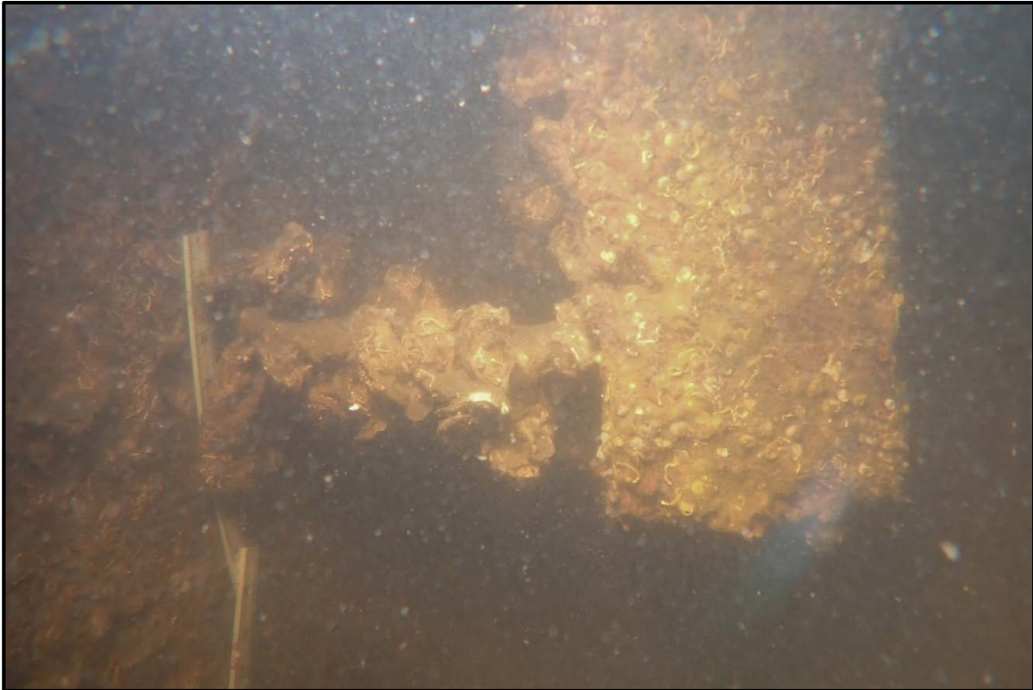
PHOTO 2-14 Aluminum alloy anode with broken lower bracket connection to sheet pile web.
