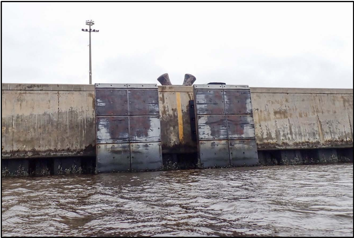
PHOTO 2-7 Typical pair of fender units.
