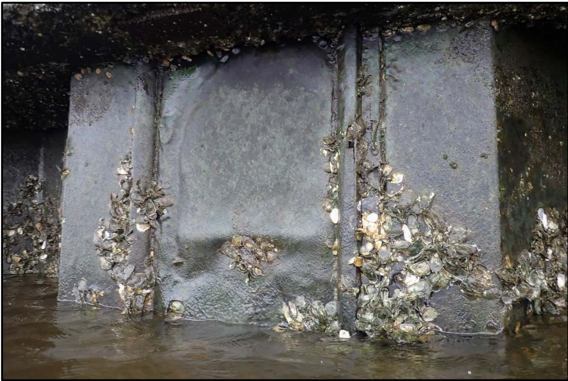
PHOTO 2-11 Delaminating epoxy coating with bubbles forming on the outer flange of the king pile.
