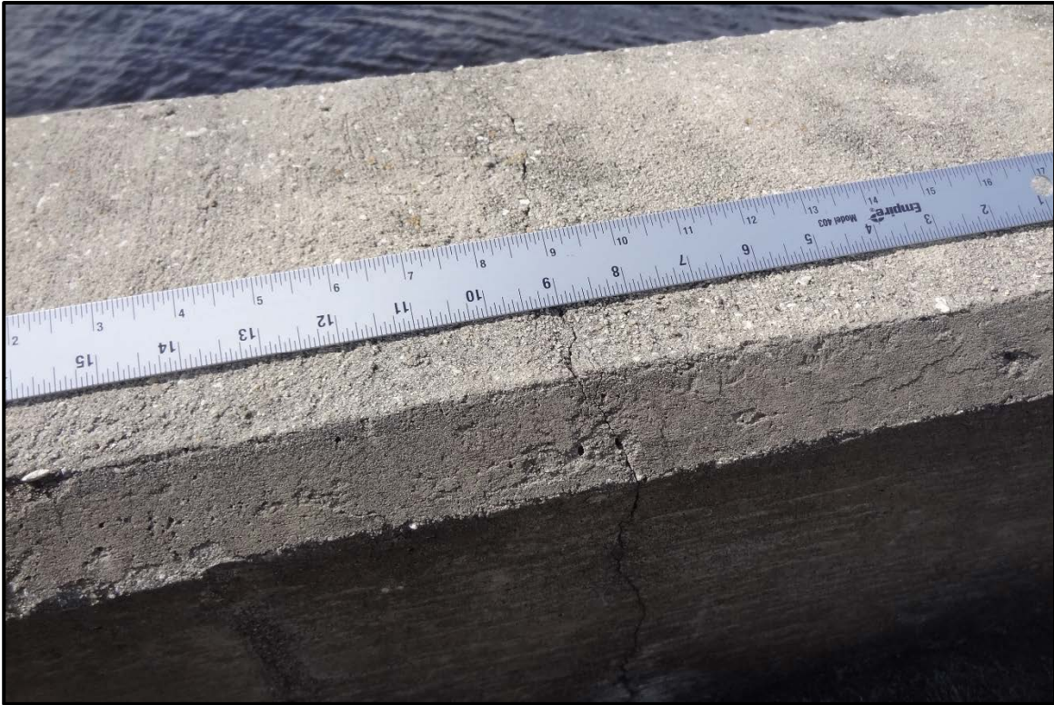
PHOTO 2-16 Typical hairline crack in concrete curb.
