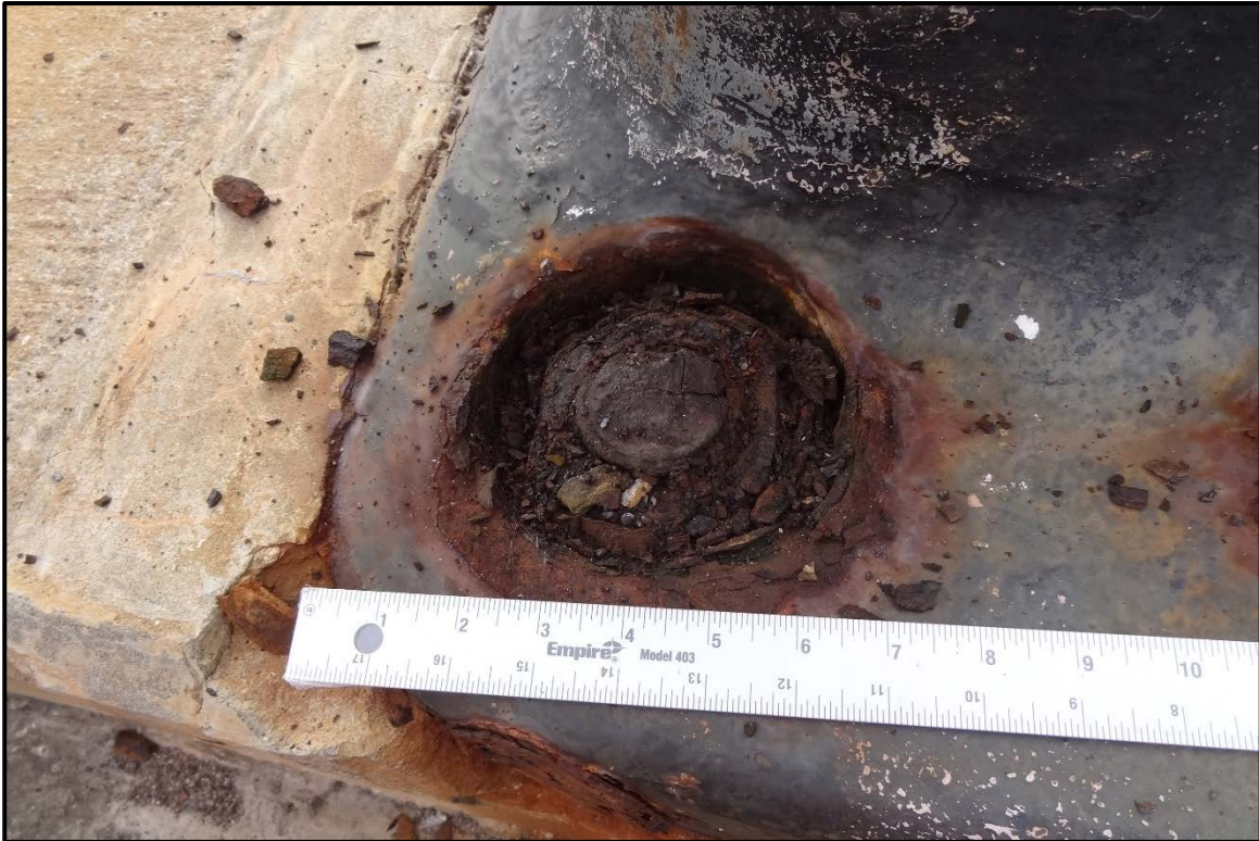
PHOTO 2-22 Exposed hardware on mooring bollard with major corrosion.
