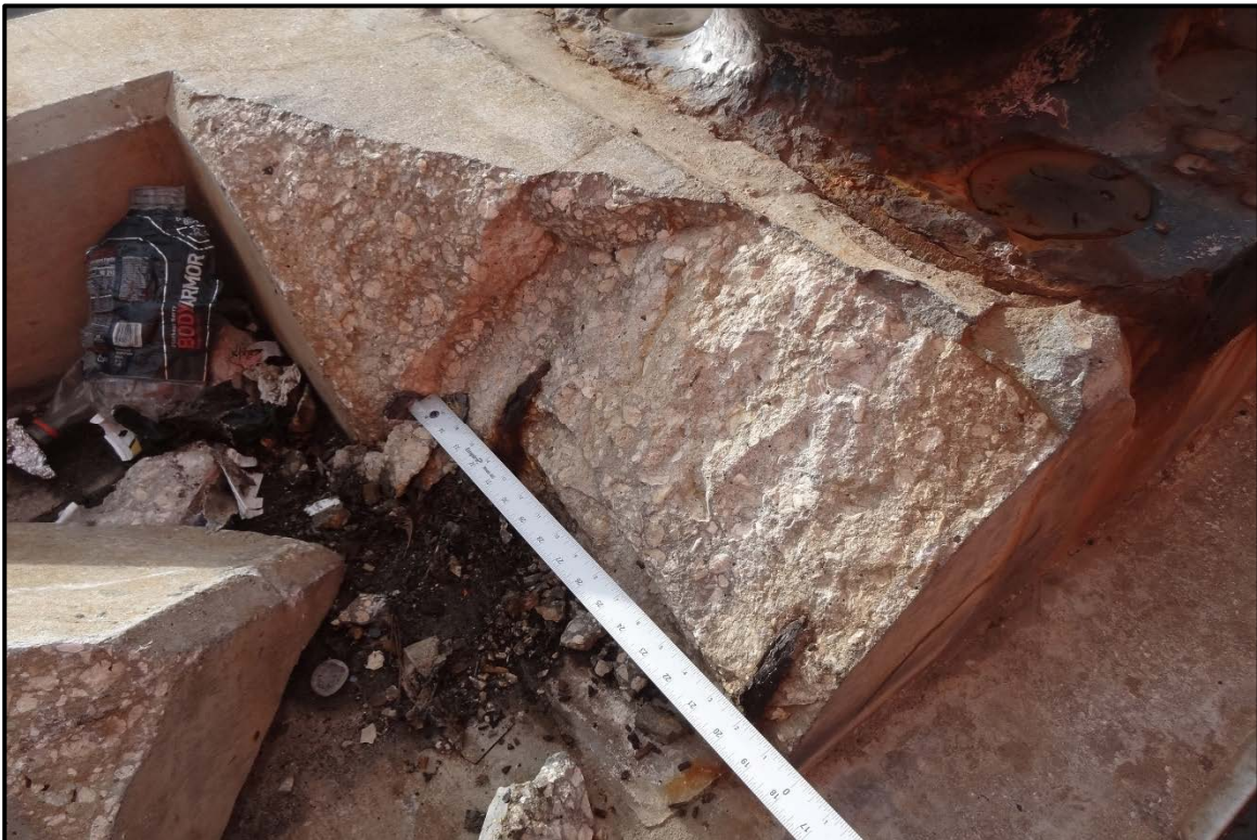
PHOTO 2-21 Mooring bollard foundation with spall exposing two reinforcing bars with severe corrosion.
