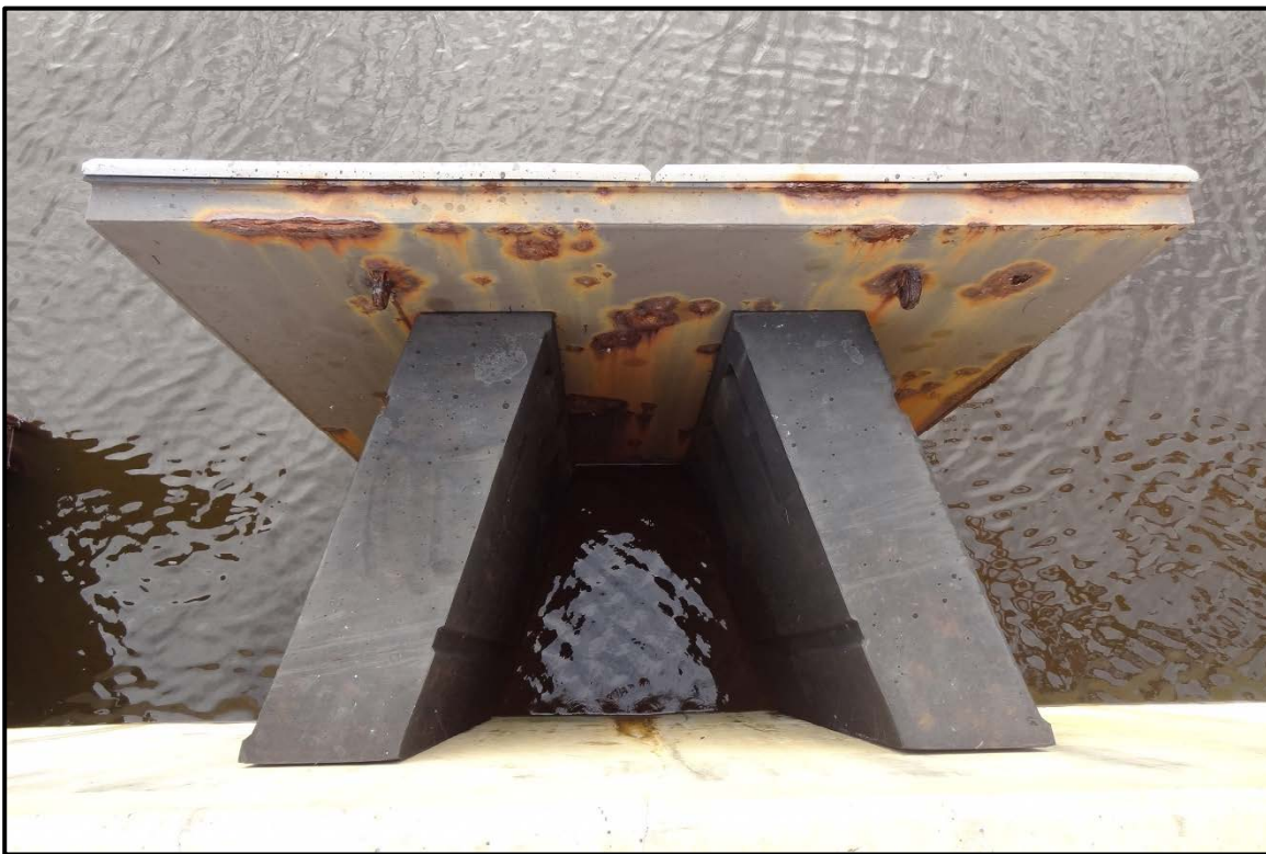
PHOTO 2-25 Typical coating loss with moderate corrosion and pitting on fender backing frame.
