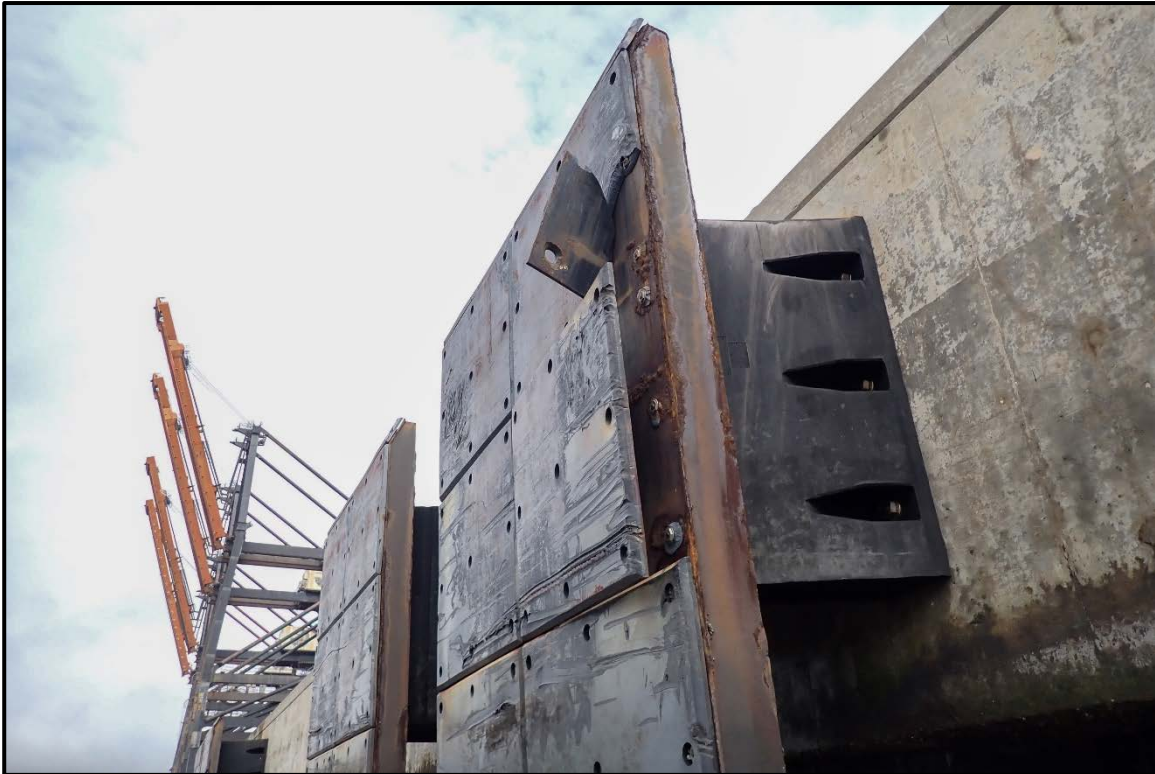
PHOTO 2-24 Loose and broken UHMW panels.
