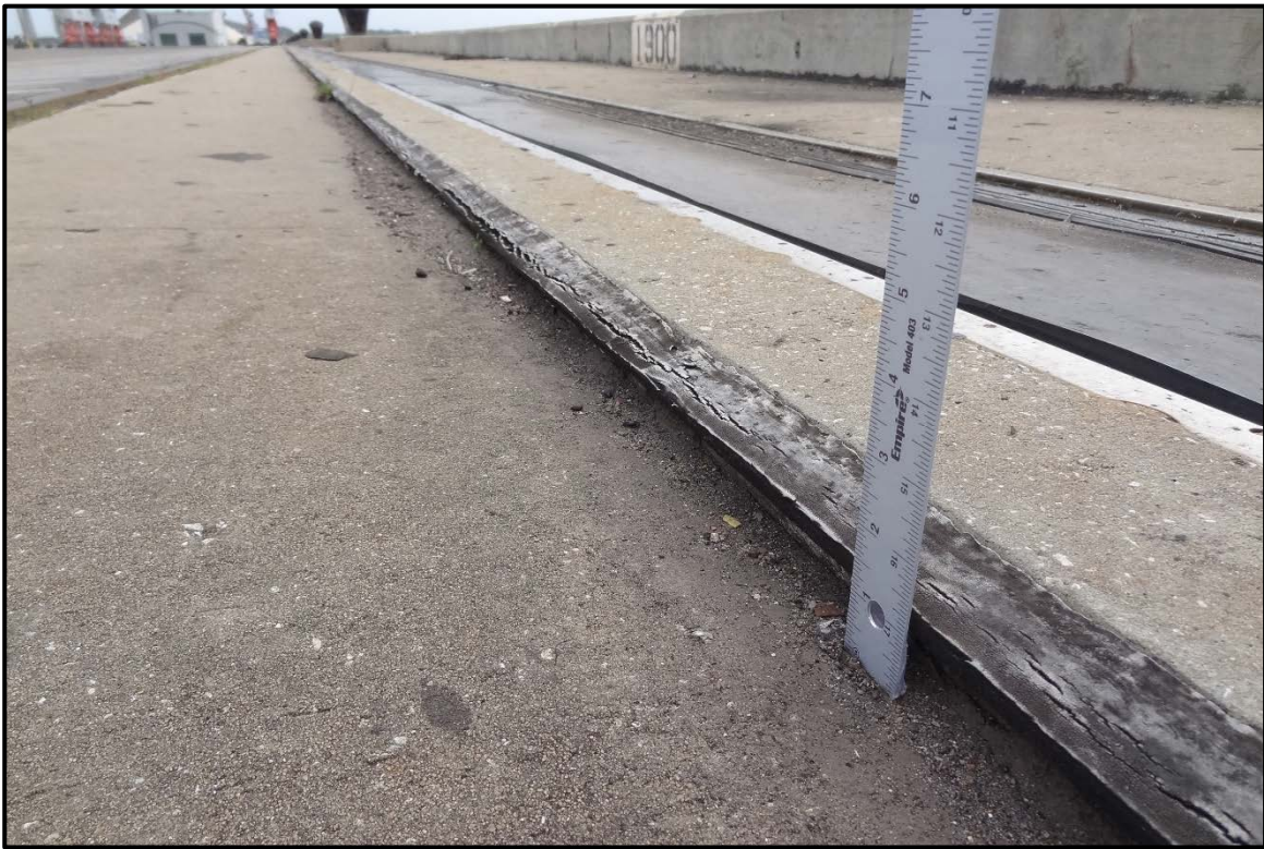
PHOTO 2-29 Differential settlement between capping beam and concrete slab located between the capping beam and crane rail beam.
