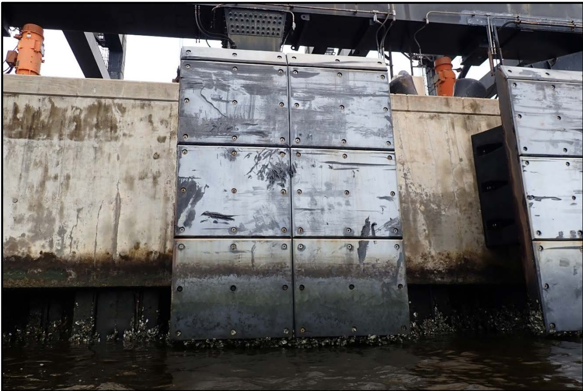
PHOTO 2-23 Typical minor cracking and gouging on the fender UHMW panels.
