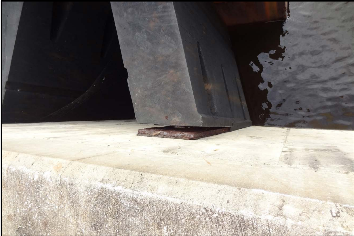
PHOTO 2-26 Rubber fender leg with crack and loose anchor bolt connection.
