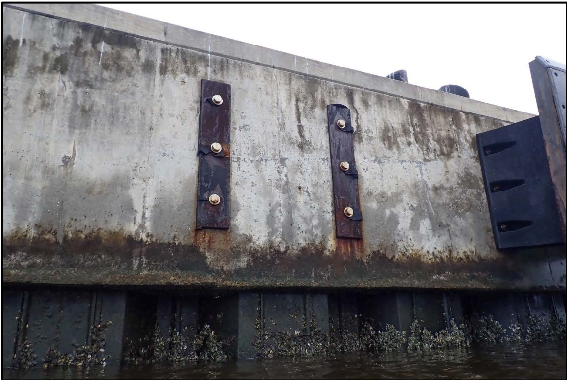
PHOTO 2-27 Missing fender unit at Station 7+80.
